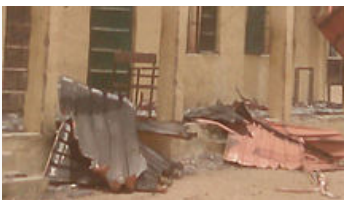
Damage to the Chibok school
